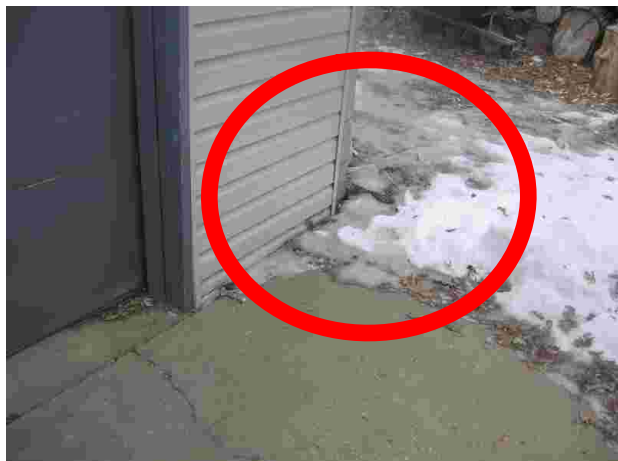
Poor drainage/low lying area at the corner of this garage.
