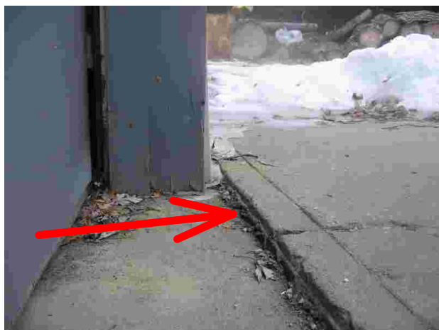
This driveway has heaved 1/2 an inch this winter due to poor drainage.
