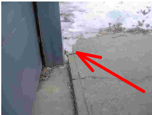
Ice showing the path of the drainage and point of entry under the driveway.
